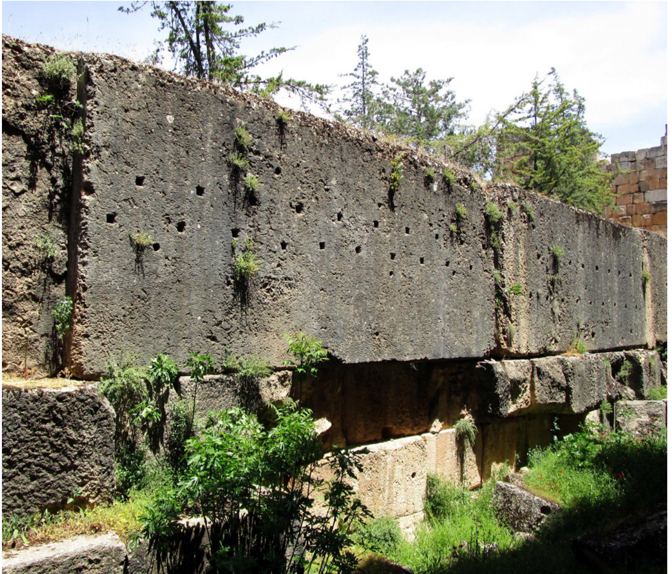
Photo. 14. Chain of plinth blocks forming the north side of the large podium, rear view. This example demonstrates that the systematically recurring “mysterious” square depressions were located not only on the front faces of the plinth blocks but also on their rear faces. The assumption that the square depressions served solely for installing anchors to secure facing slabs cannot be considered correct, since the rear sides of the plinth blocks were hardly intended to be clad. The masonry is laid with gross violations of the bonding rule; in addition, there is a section of a stretcher course laid with headers. Photo 2019 from wikimedia.org.
