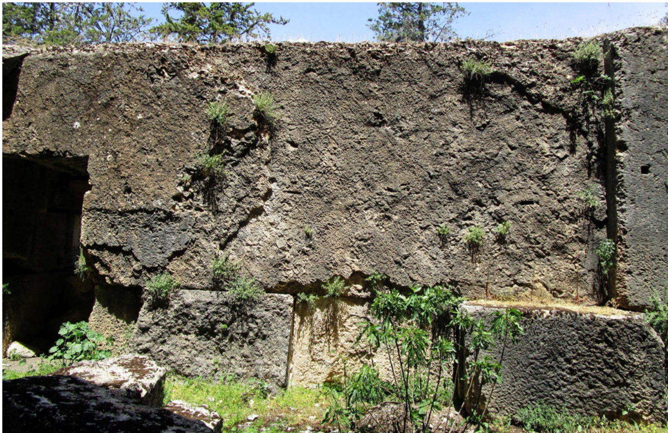
Photo. 16. Rear face of one of the plinth blocks on the north side of the large podium. The outer vertical concrete wall of this face has almost completely collapsed. The coarse gravel aggregate in the concrete filler did not settle at the bottom of the wall during pouring; instead, it is distributed more or less uniformly across all heights. On the left, where the wall has not yet fully collapsed, the remnants of square depressions are visible. The absence of the square depressions on the remaining surface indicates that their depth was equal to the thickness of the outer concrete layer of the wall. Photo 2019 from wikimedia.org.
