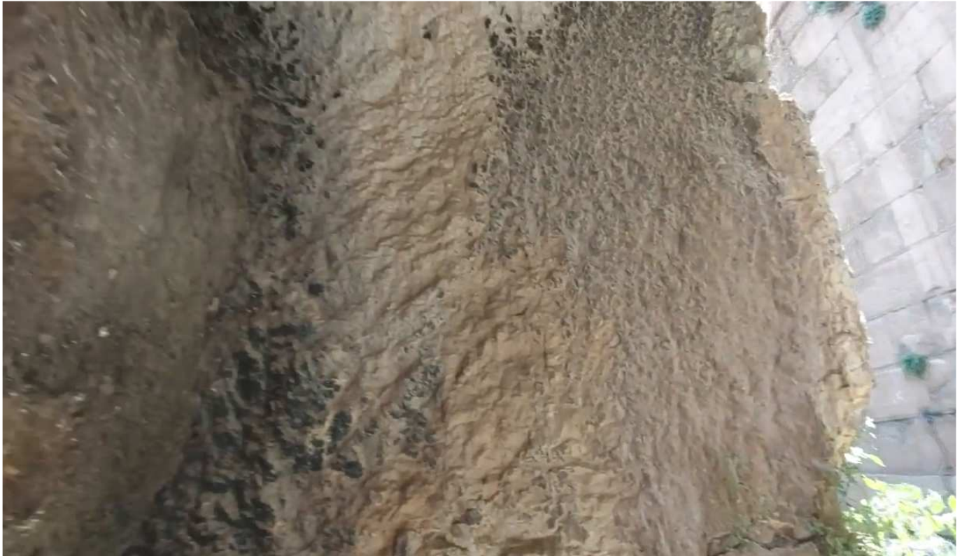
Photo. 17. Cross-sectional view of the plinth block from the side of the passage left by the builders. On the right, along the edge, remnants of the collapsed outer concrete wall are located; in the center – the internal concrete longitudinal partition. The darker areas to the left and right of the partition represent the internal masonry of stone blocks, which serve as a solid filler. Frame from the video “Showing inside the “megafence” of Baalbek”, 2023.
